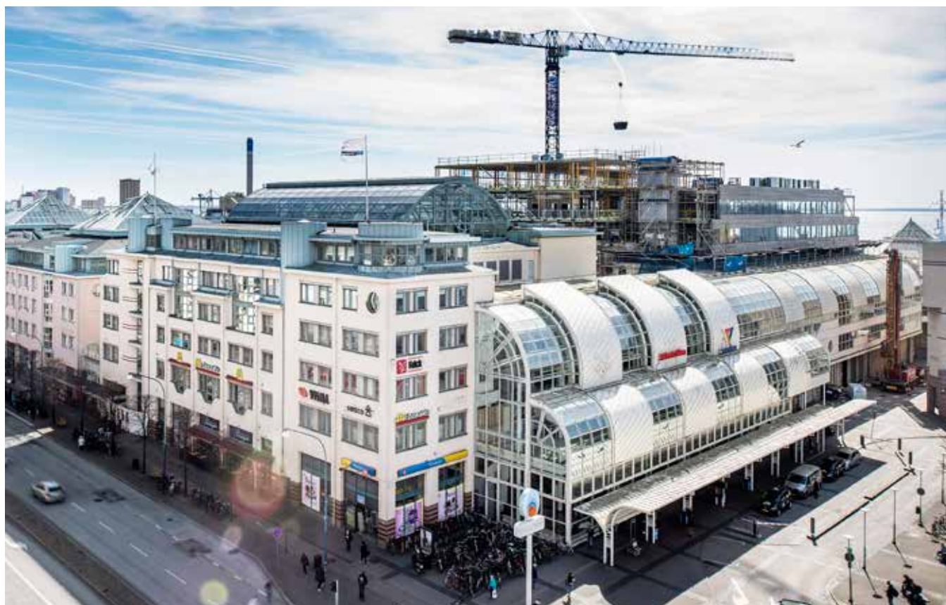
At Knutpunkten in Helsingborg, the new extension is taking shape and facade sections are starting to appear. In the first phase, 7,700 m 2 of offices are being built with views of the sound and the city-centre roofline. Future phases will include a rebuild of the transport hub.
