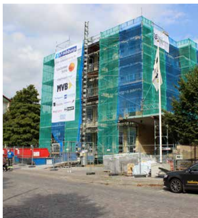
Wihlborgs is renovating the Landstinget 2 building in Lund on behalf of Sparbanken Skåne. The project is due to be completed on 1 January, 2015.
