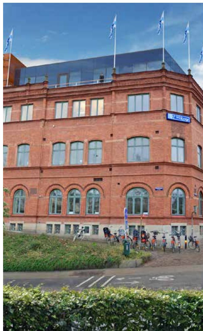
A 1,000 m 2 extension is being built at roof level on the Armaturen 4 property, creating superb offices with views over Lund.
