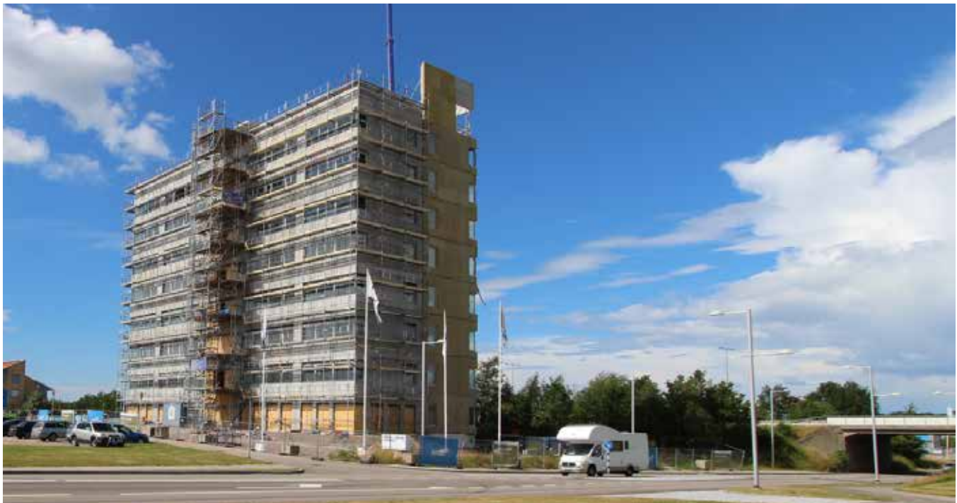
The tallest building at Berga, Helsingborg, reached its full height in June. It is estimated that Floretten 4 will be complete by year-end.
