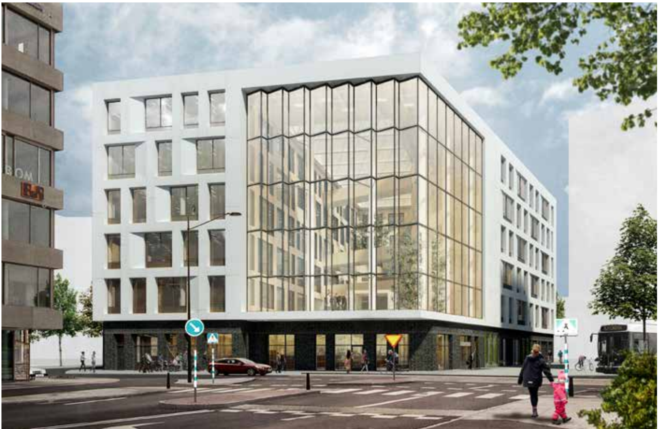
In Hyllie, Wihlborgs is building the Dungen office building on the Gimle 1 site. Swedish Customs has signed a lease for 6,300 m 2 with occupancy planned for the first quarter of 2019.
